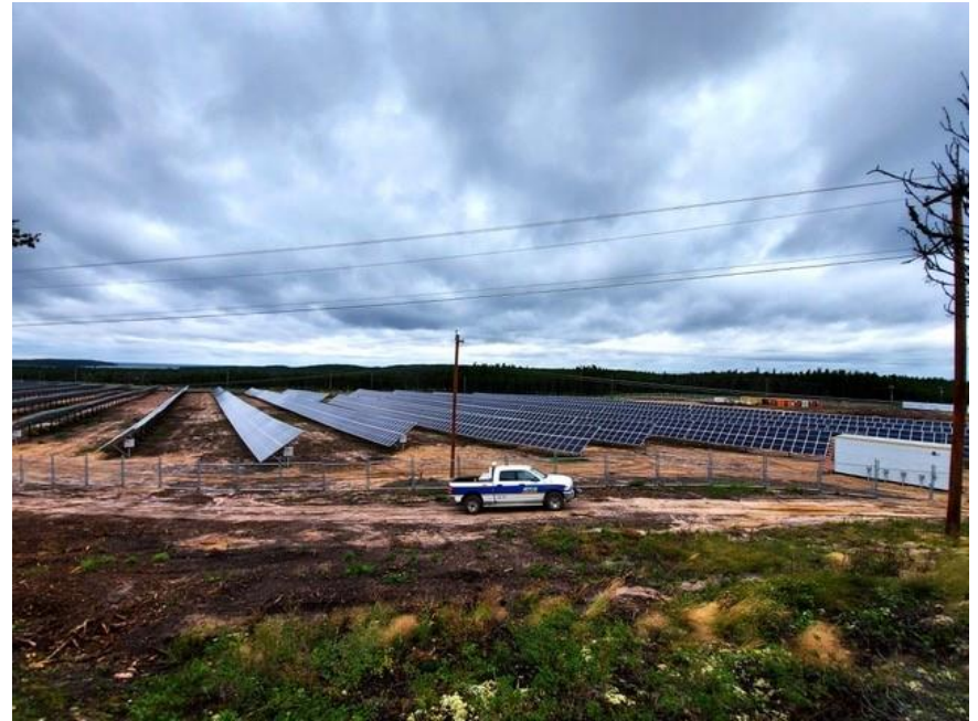
ATCO's Fort Chipewyan Microgrid Energy Storage Project
